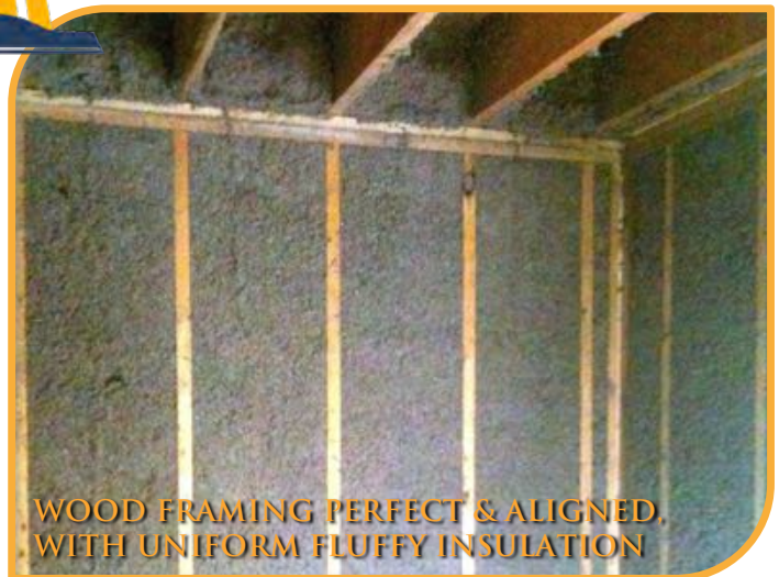
TOO MUCH WOOD, TOO LITTLE INSULATION CRAMMED IN
