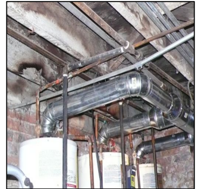
Major moisture damage over water heaters
