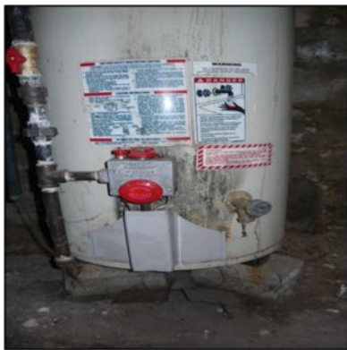
Water heater shows signs of flame roll-out
