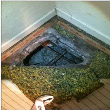
Crawlspace under the carpet- major issue
